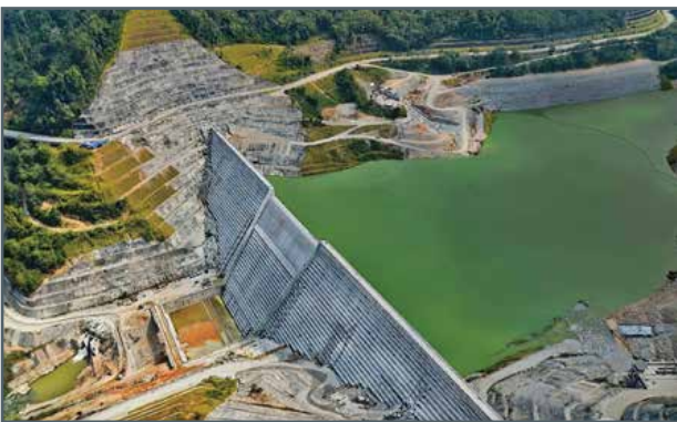
The Ulu Jelai Dam, Malaysia. Owner-Tenaga Nasional Berhad. Constructor- Salini. Systems - Maxwell GeoSystems.
